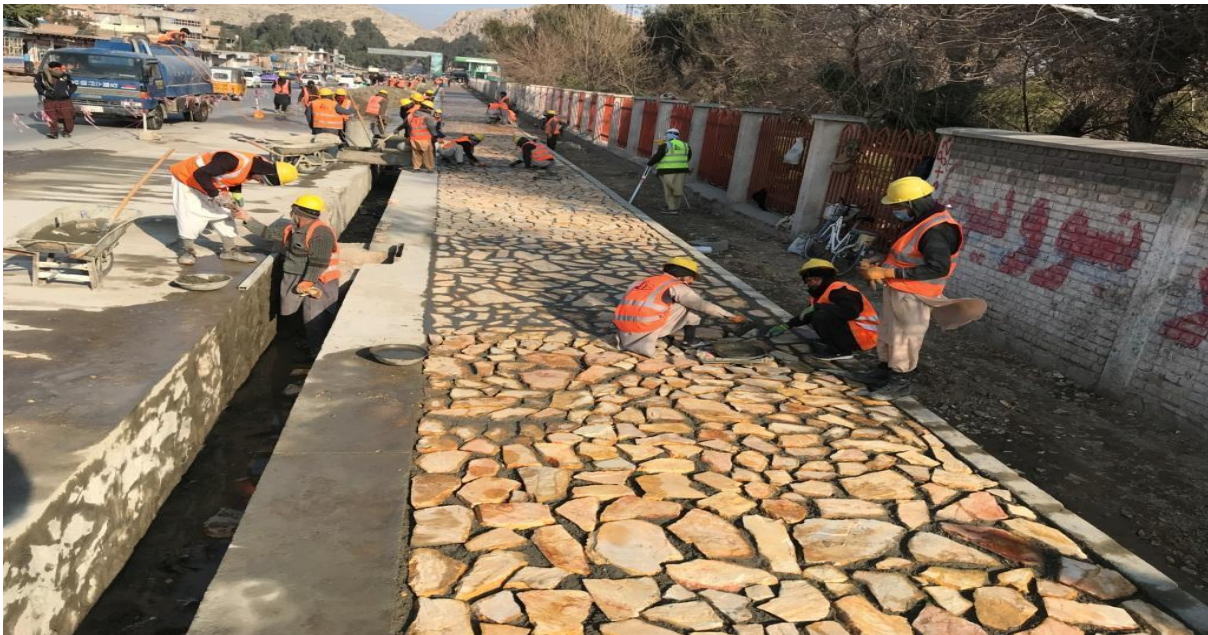
Photo: Stone patching and PCC work is in progress in front of Nangarhar University, District-7 of Jalalabad city on 18 Dec 2022
