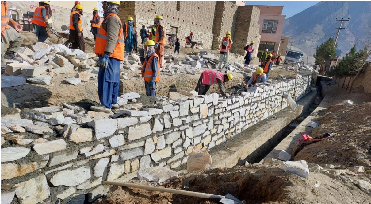
Photo: Construction of stone masonry wall of Khairabad Chaman Street and side drains, District-20, Kabul City on 27 Dec 2022
