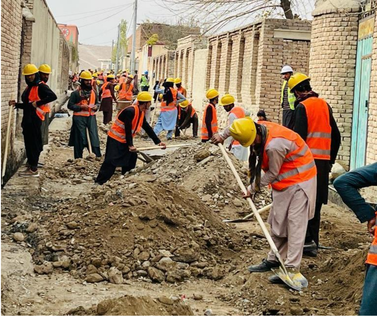
Photo: Excavation activities for Matoon Wrgaha to Prison in Sarankoot main road, District-5, Khost Province
