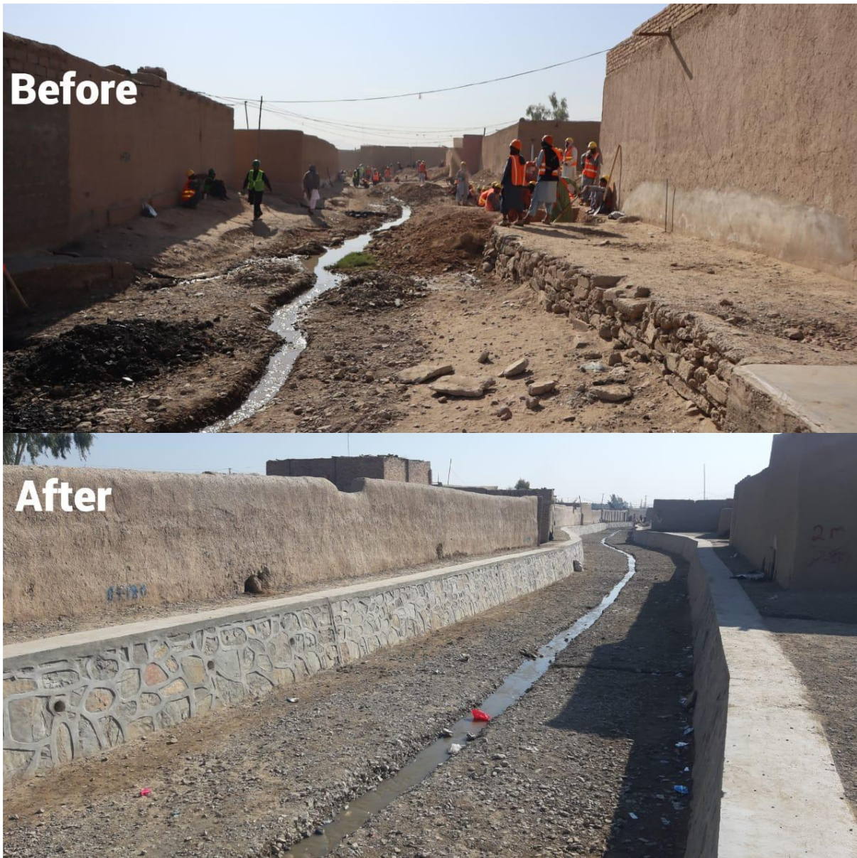
Photo: Before and after condition of Protection Wall for Sahil Drainage Channel, Dist#12 of Kandahar city
